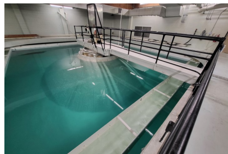
Softening Clarifier at ELMWSA
