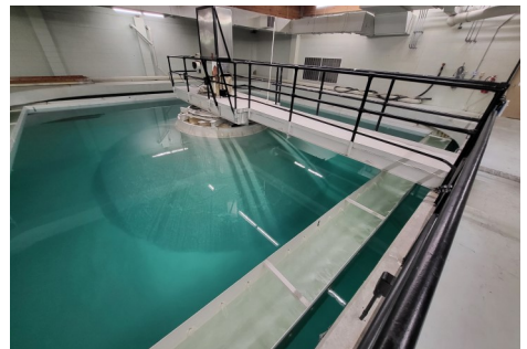
Softening Clarifier at ELMWSA
